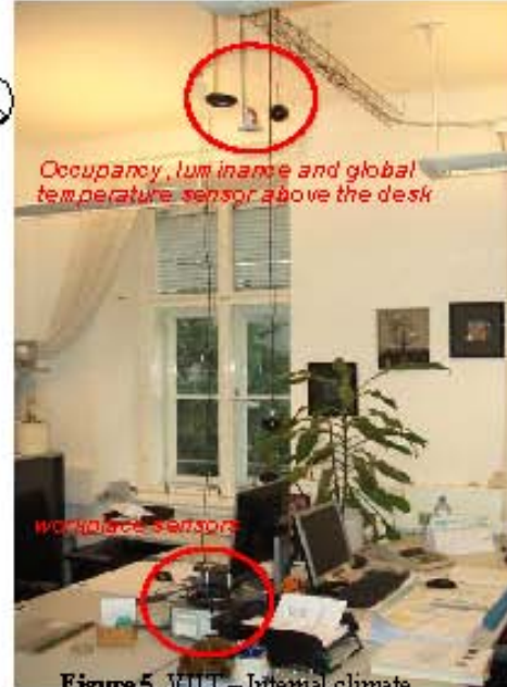
Figure 5. VUT – Internal climate sensors
